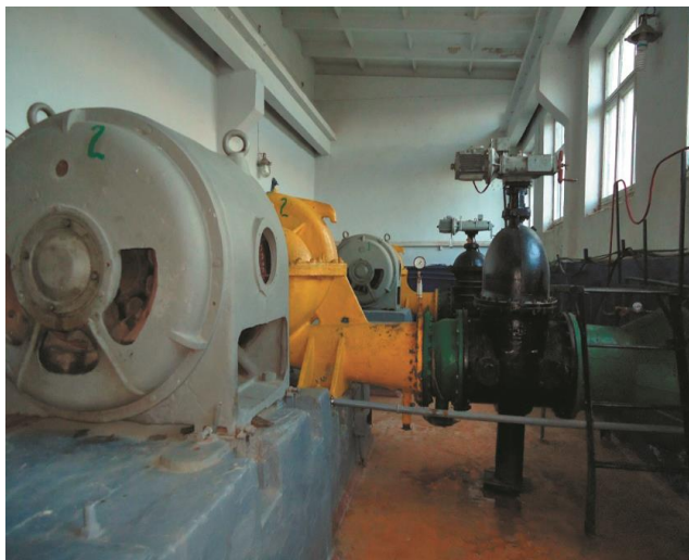
Fig. 1.18. Technical equipment for adding coagulants (photo by Marina Ilyasova).
