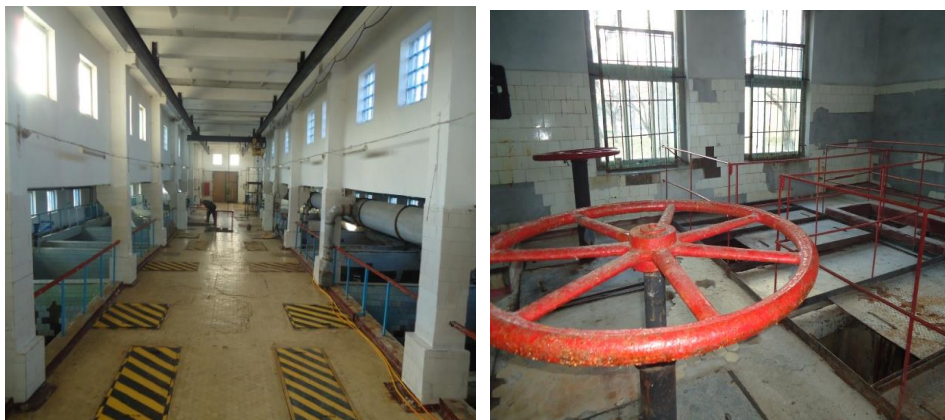
Fig. 1.16. Mesh chambers where filtration takes place – the first stage of water treatment (photo by Marina Ilyasova).
