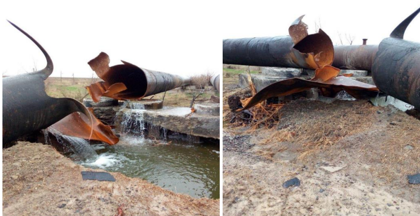
Fig. 1.19. Damaged water pipeline "Dnipro-Mykolaiv" on the territory of the Kherson region, 2022 (photo from open sources)
