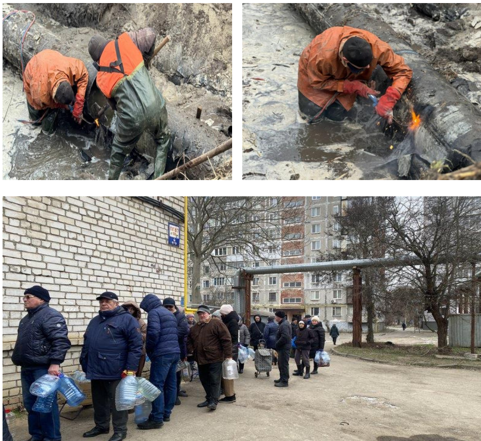
Fig. 1.35. While repair work is being carried out on the duker, people are standing in queues for water (photo from open sources).
