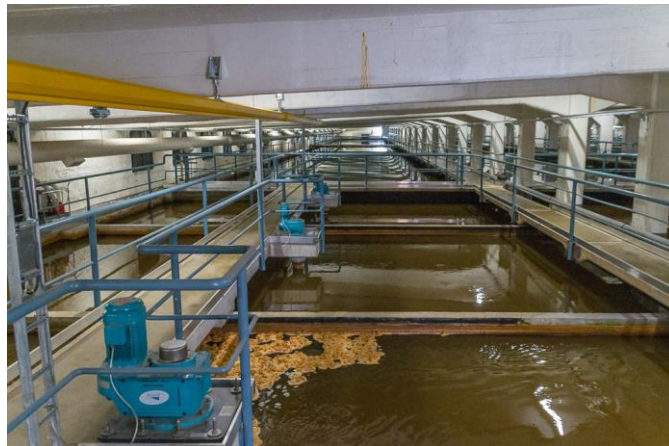
Fig. 4.11. View of coagulation & flocculation process in real waterworks.
