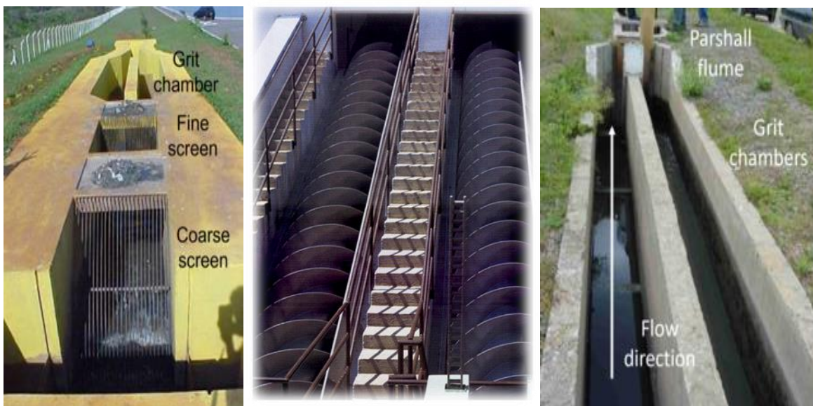
Fig. 4.17. Manually-cleaned screens (left); sewage pumping into the next technology units of wastewater treatment plant (middle); horizontal flow grit chambers (right).
