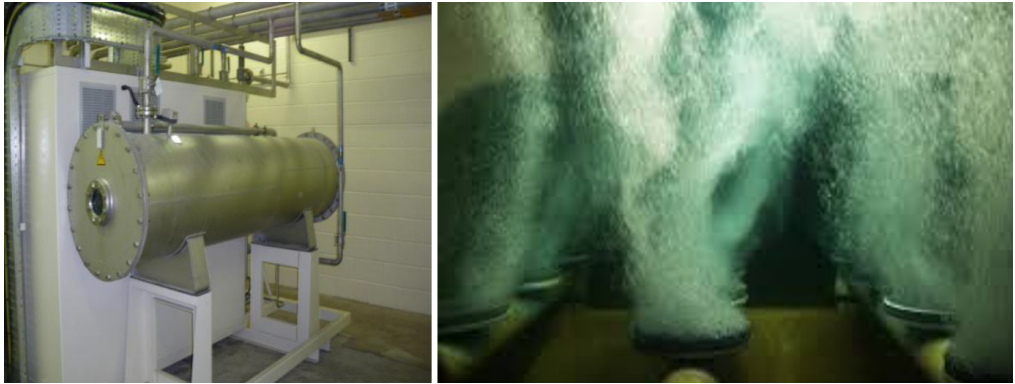
Fig. 3. Ozone bubblers in operation at Purton WTW (Source: Bristol Water)
